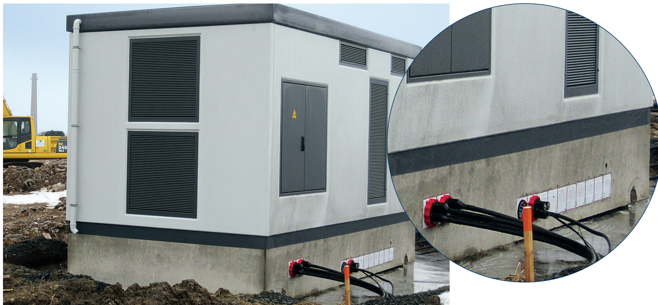
Transformer station of an onshore wind power station: the cables have been sealed with a HSI 150 packing piece using various system covers.
